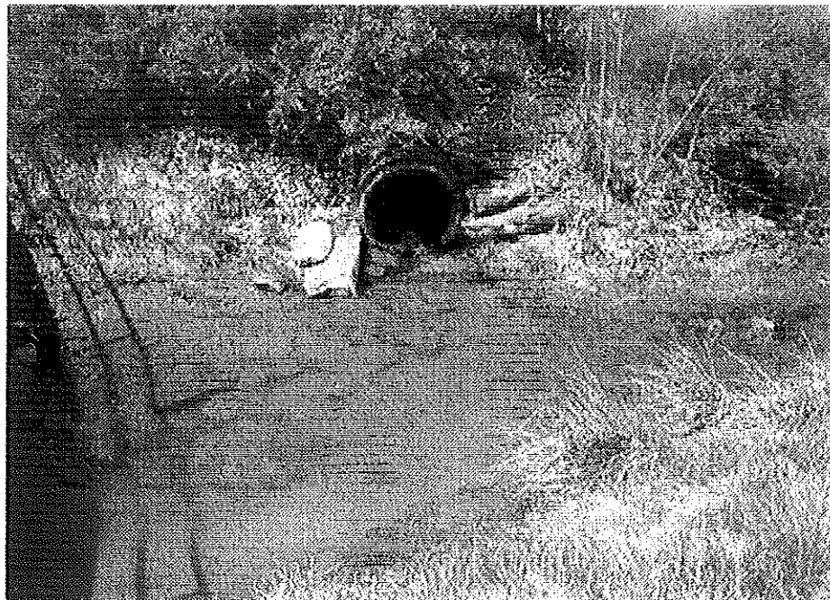
Figure 3. This picture shows the first pipe which is located at the end of site #1.
